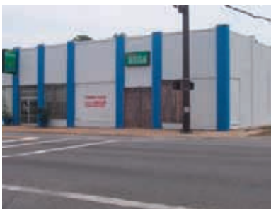
Vacant and Boarded Structure along Pace Boulevard
