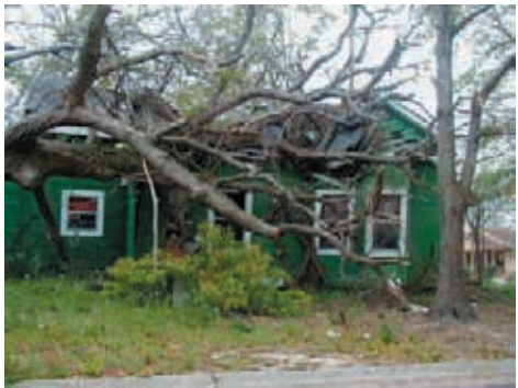
Derelict House: I Street
