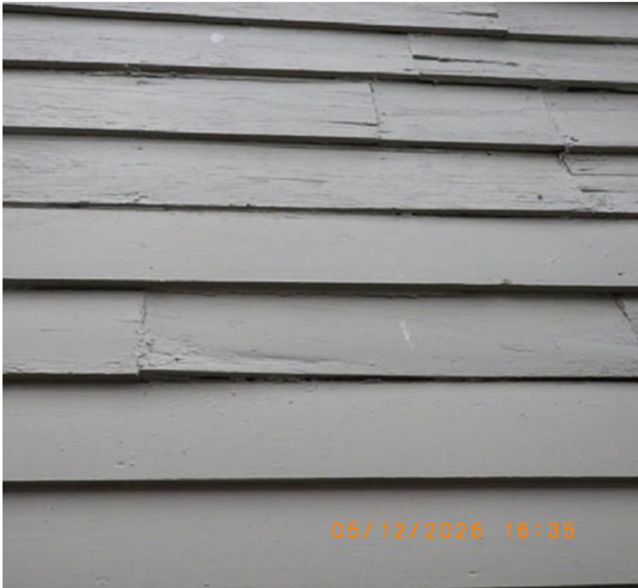
Damaged Existing Siding
