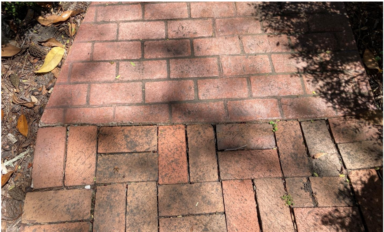
Photo 12: Two different walkway types: wire cut clay brick (Glen Gery Full, Range 2-1) and stamped concrete with brick pattern. The concrete sidewalk cracked and sections lifted from tree roots.
