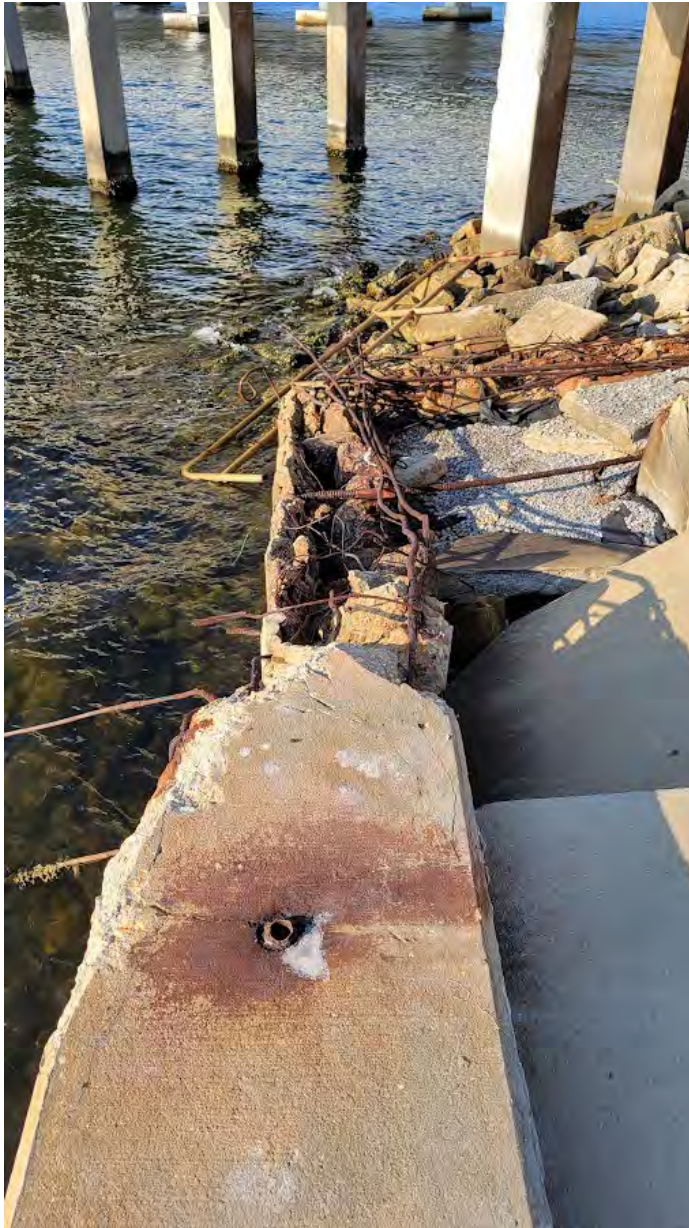
Photo 1: Damaged southernmost bulkhead
