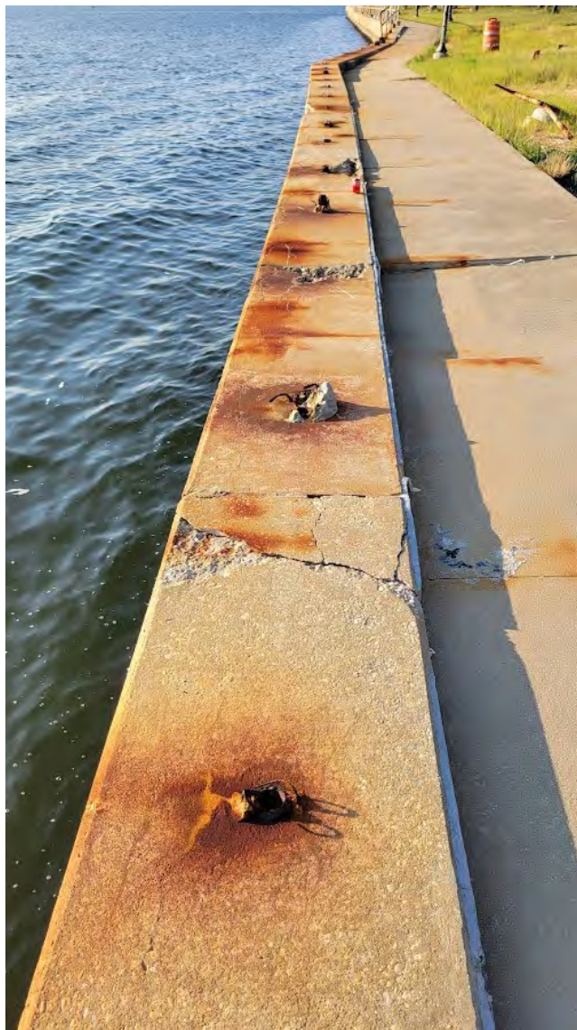
Photo 6: Damaged cap, handrail, and sidewalk collapse.
