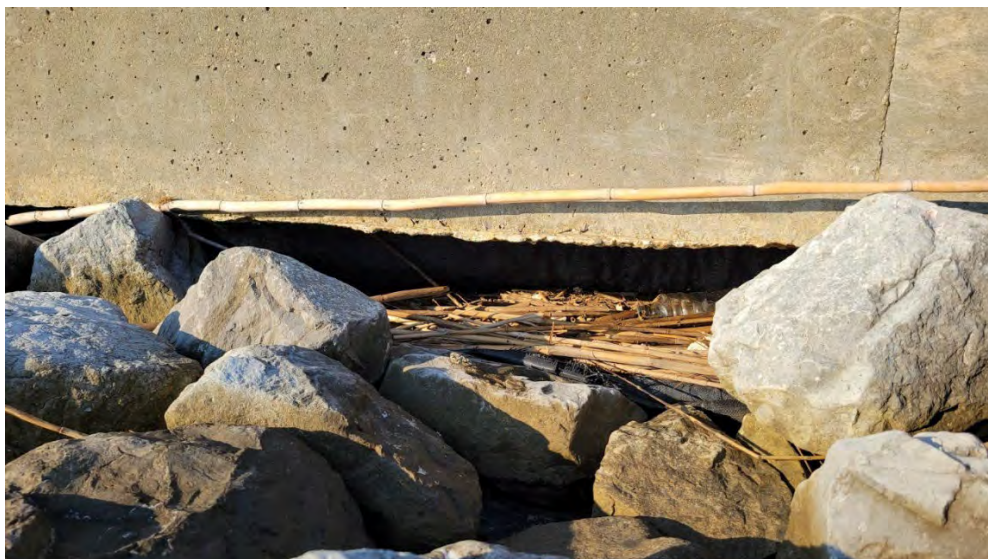
Photo 9: Undermined ground-supported beam at revetment
