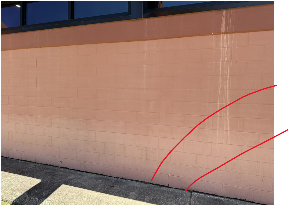
Photo 20 – West Exterior Wall (Looking East; Stair Stepped Cracking)
