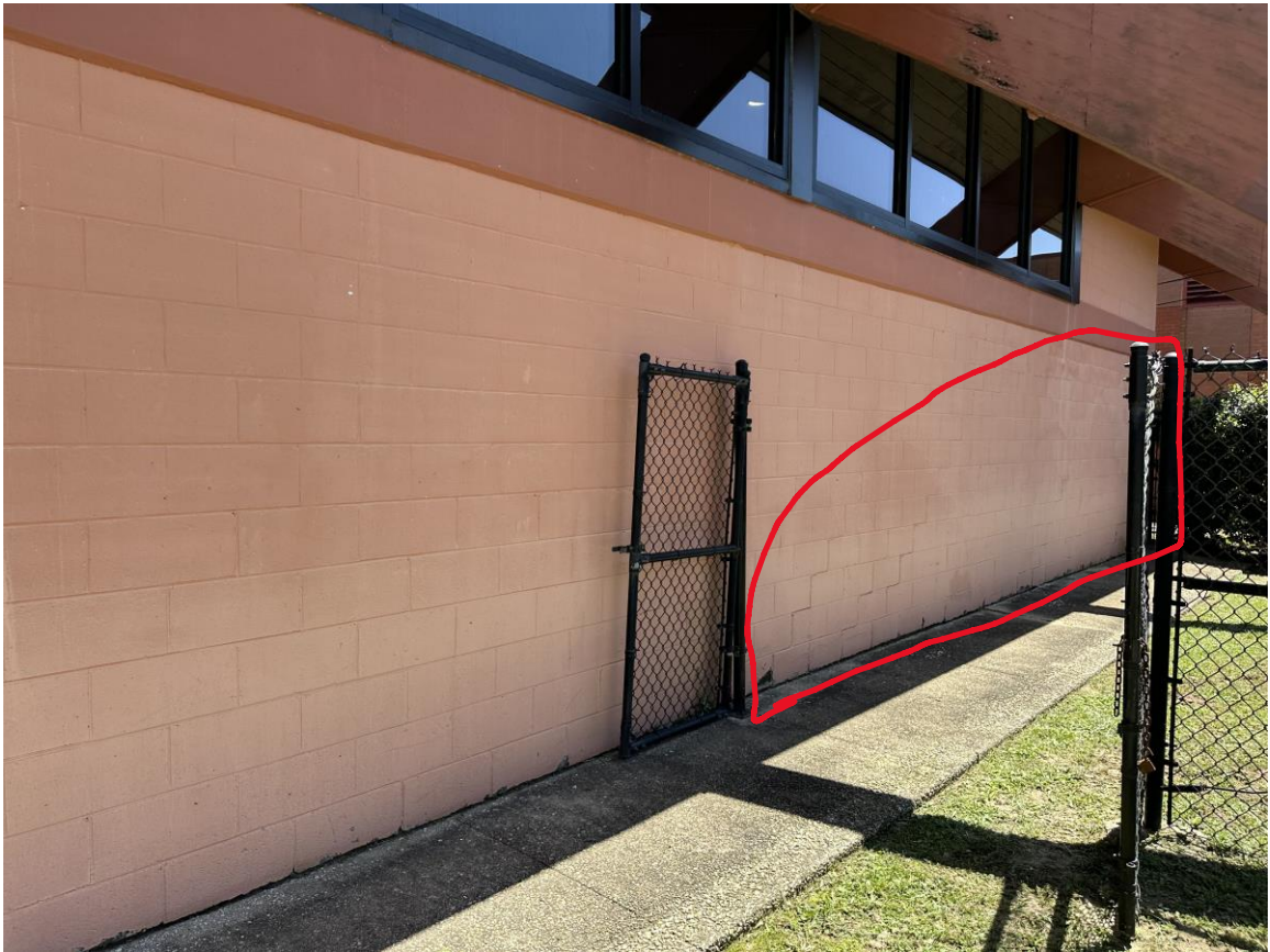
Photo 22 – West Exterior Wall (Looking Southeast; Stair Stepped Cracking)
