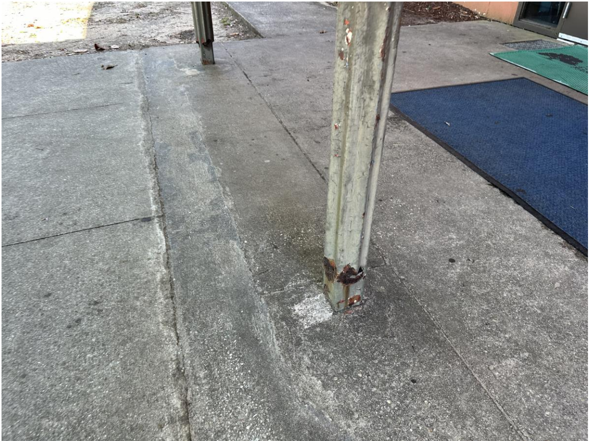
Photo 14 – North Entrance Canopy (Corrosion at Steel Support Columns)
