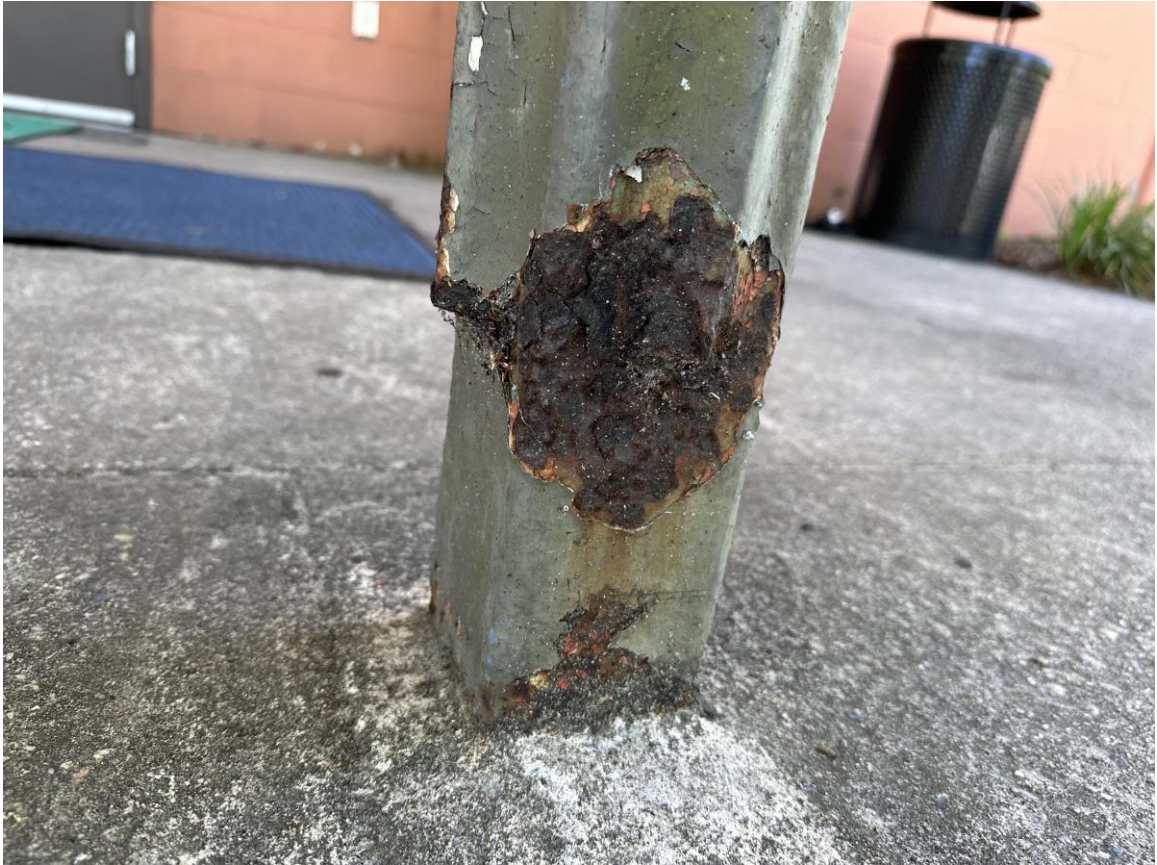
Photo 15 – North Entrance Canopy (Corrosion at Steel Support Columns)
