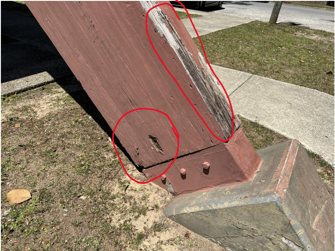
Photo 4 – East End of North Arch (Decay)
