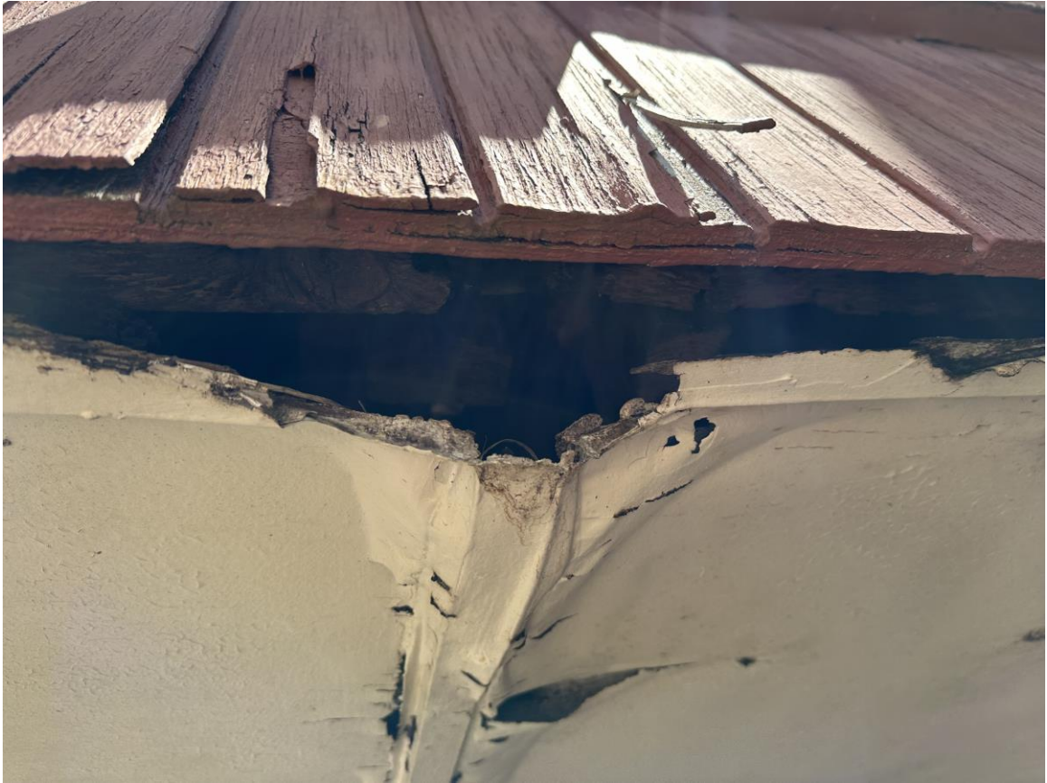
Photo 11 – North Entrance Canopy (Soffit & Roof Framing Water Damage)
