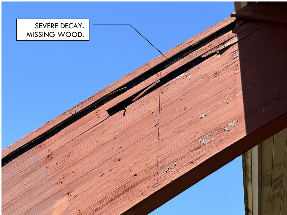
Photo 9 – West End of Arch (Decay)
