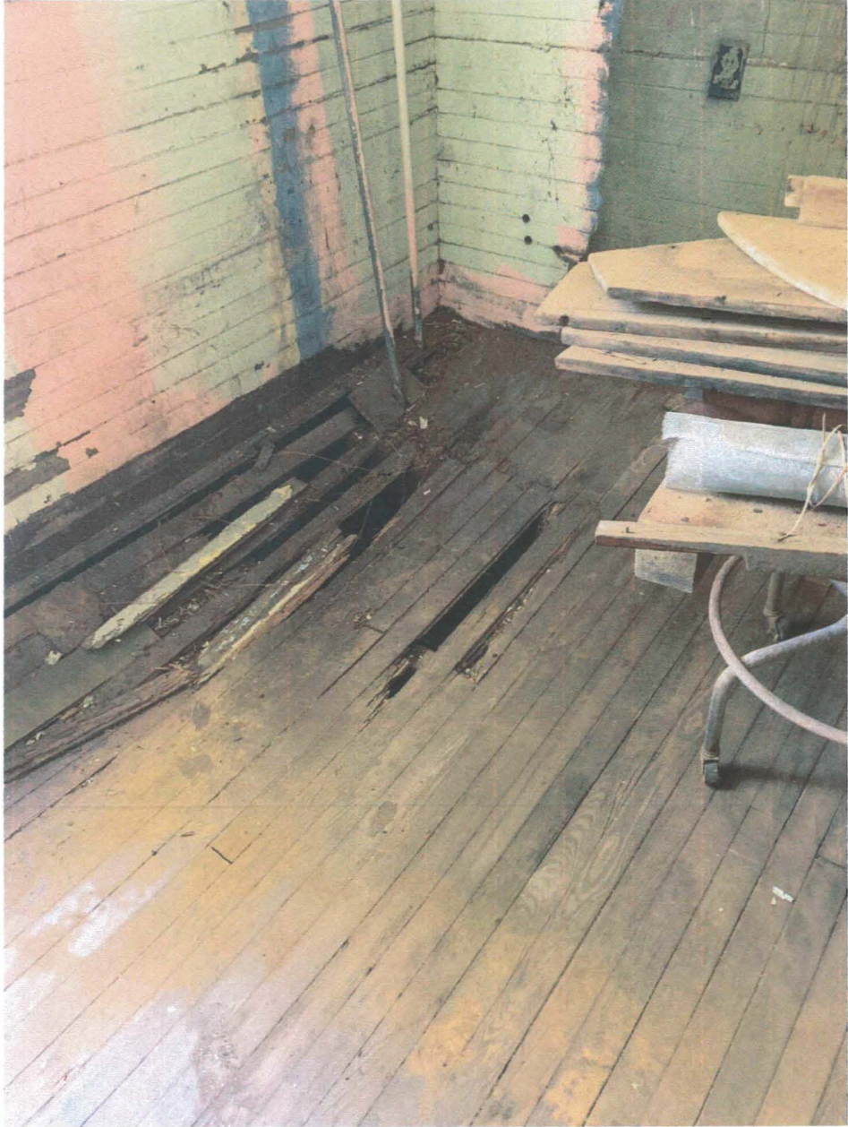
Floor Condition, in Old Kitchen to be Demolished
