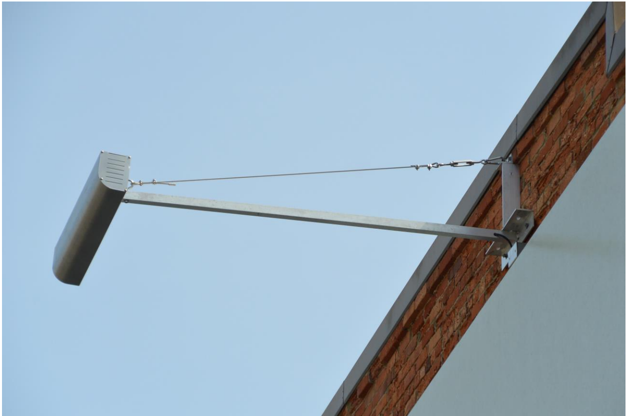
Overhead mounted LED 150 watt light for each panel. Light shown is located above the existing wallscapes on the Voices of Pensacola building and the Museum of Commerce.
