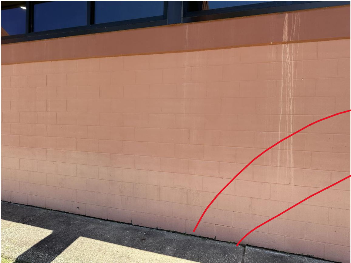
Photo 20 – West Exterior Wall (Looking East; Stair Stepped Cracking)
