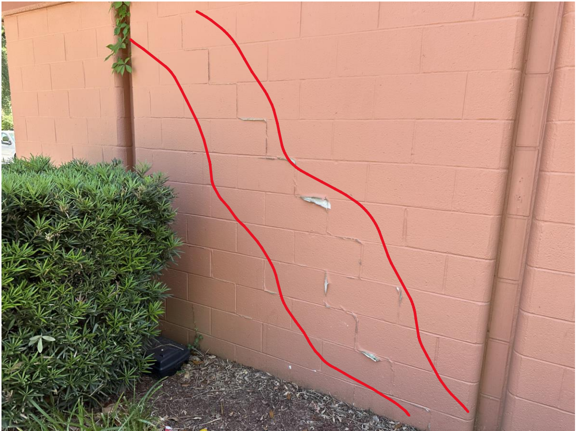
Photo 17 – North Exterior Wall (Stair Stepped Cracking at East End)
