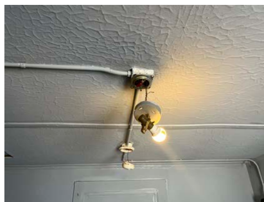
Damaged Fixture Example
