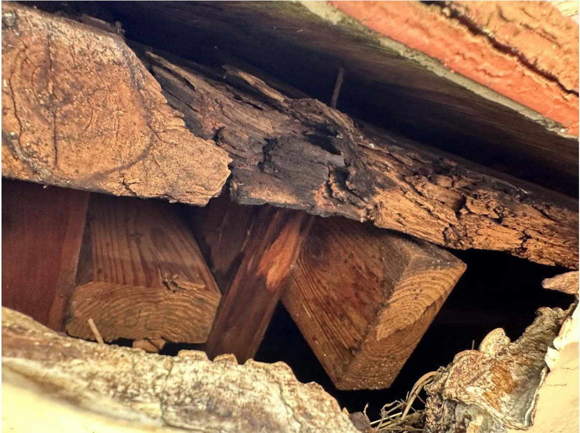
Photo 12 – North Entrance Canopy (Soffit & Roof Framing Water Damage)
