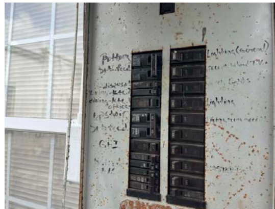
Building #11 - Electrical Panel
