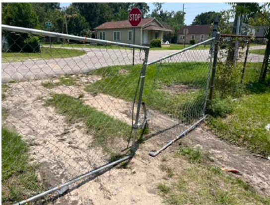
Chain Link Fence Damaged Gate
