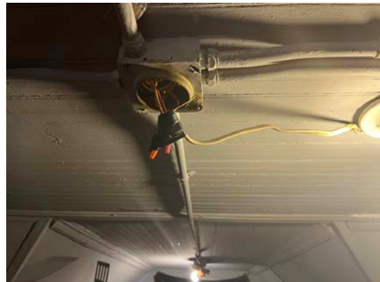
Building #2 Attic Space - Missing Fixture
