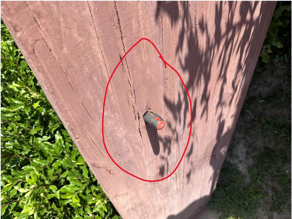
Photo 7 – Southernmost Arch on West Side (Decay Depth is ~7")
