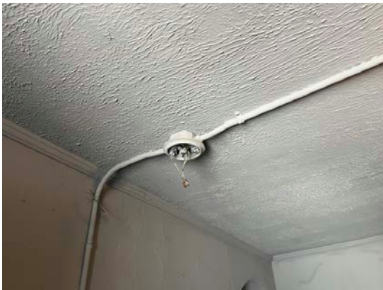
Missing Smoke/CO2 Detector
