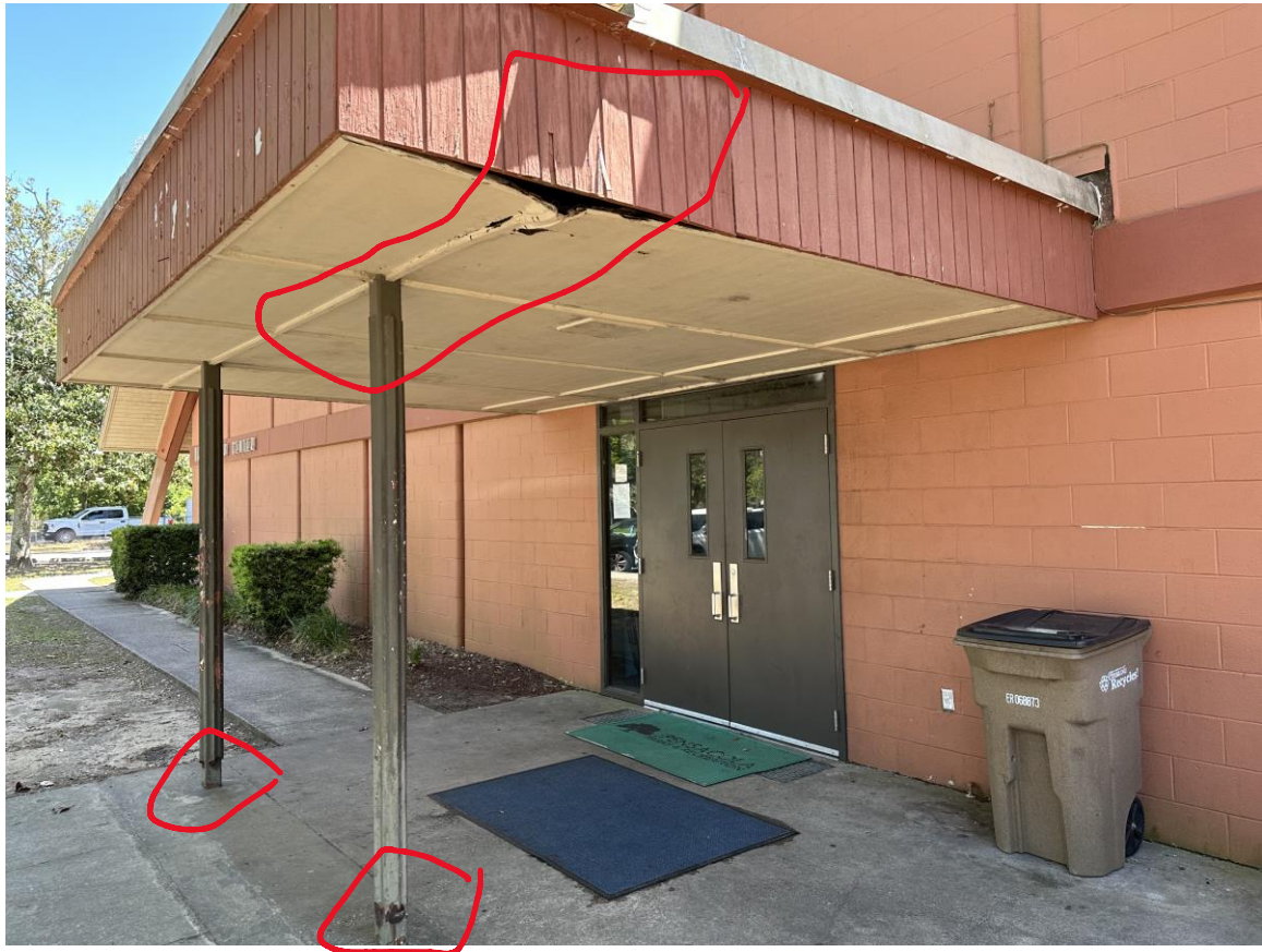
Photo 10 – North Entrance Canopy (Water Damage)
