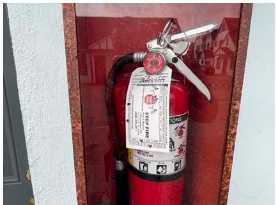
Common Area Fire Extinguisher
