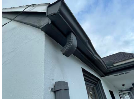
Disconnected Downspout and Damaged Gutter
