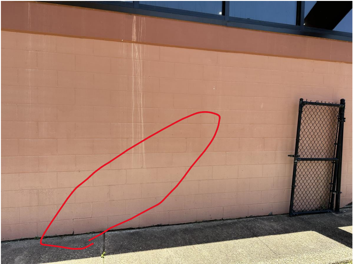
Photo 21 – West Exterior Wall (Looking East; Stair Stepped Cracking)
