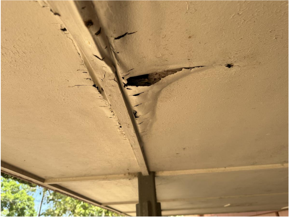
Photo 13 – North Entrance Canopy (Soffit & Roof Framing Water Damage)
