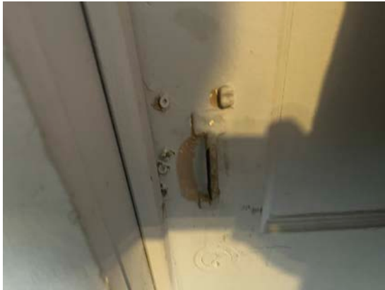
Unit Water Heater Closet - Room Not Accessible Example
