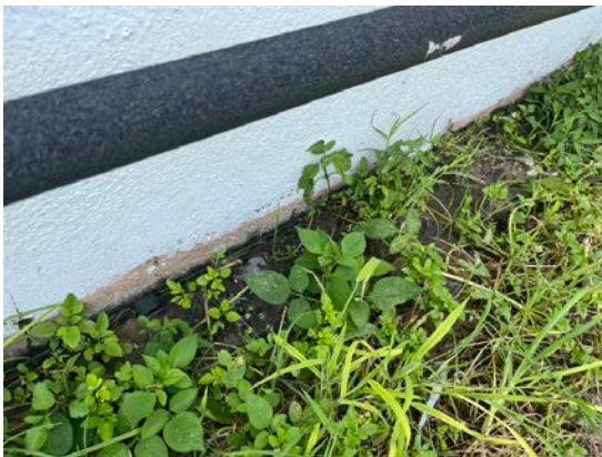
Water Ponding From AC Drain - Building #2
