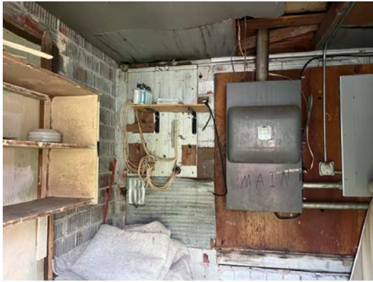
Electrical Service Administrative Building
