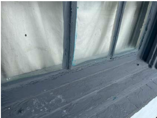
Unit Window - Painted Closed
