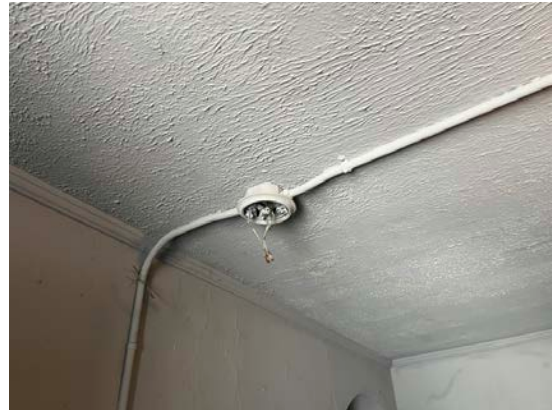
Unit #114 Light Fixture
