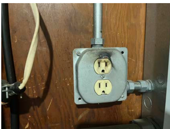
Burned Outlet - Building #6
