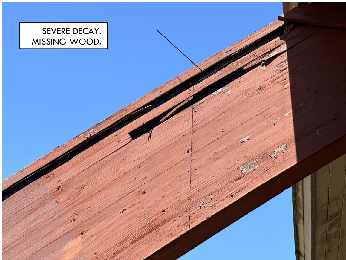
Photo 9 – West End of Arch (Decay)
