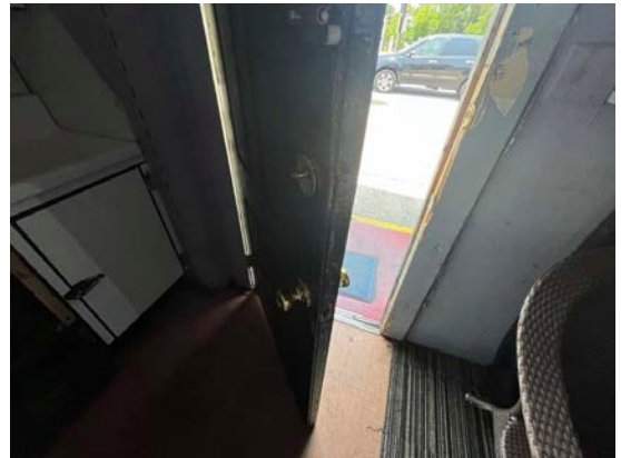
Unit Entry Door and Broken Frame
