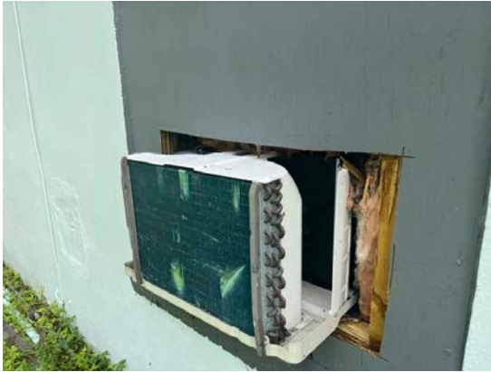
Broken AC Unit - Example
