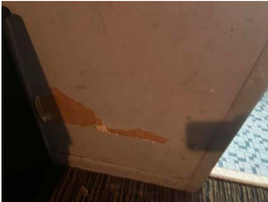
Unit #103 Interior Wall Damage
