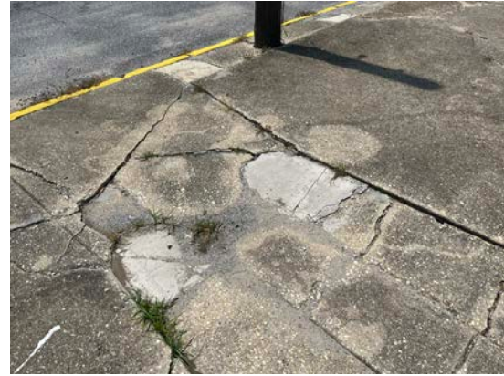
Broken Concrete Parking Island
