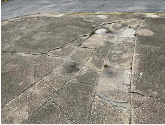
Broken Concrete Parking Island
