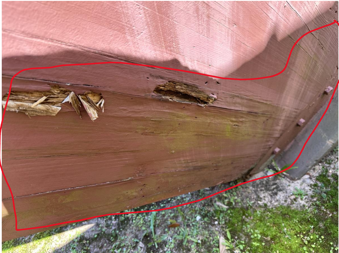
Photo 5 – East End of Center Arch (Decay)
