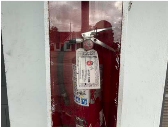
Common Area Fire Extinguisher
