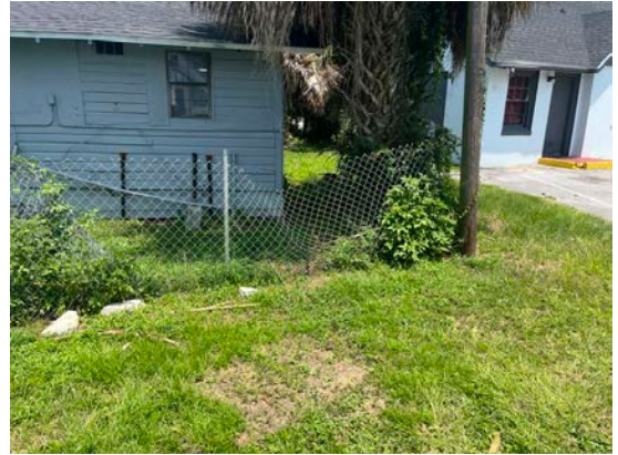
Chain Link Fence Damage Example
