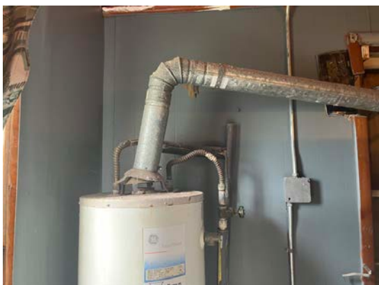
Laundry Room Water Heater
