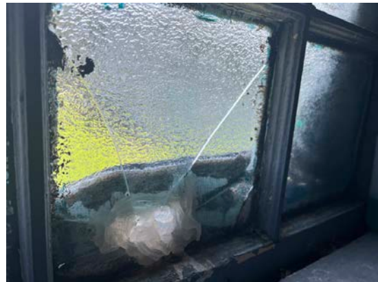
Unit Window - Broken Glass
