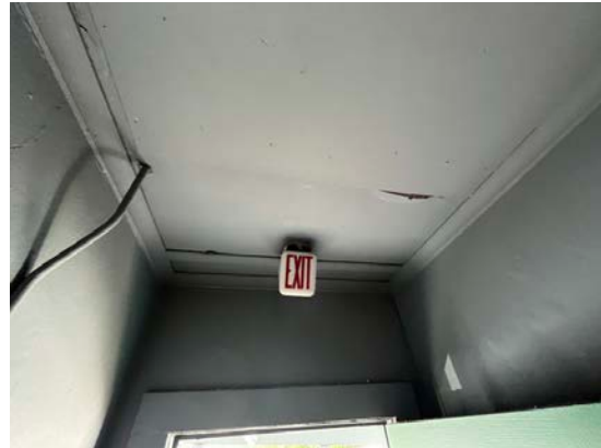
Emergency Exit Signage
