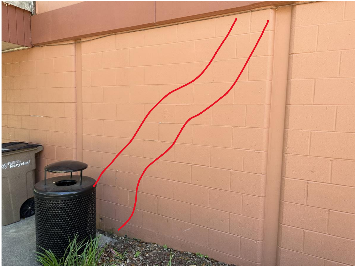
Photo 18 – North Exterior Wall (Stair Stepped Cracking West of Door)
