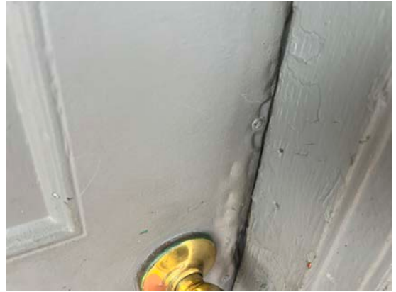
Unit Entry Door - Damage and Repair
