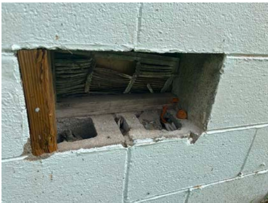
Missing CMU Block - Building #7
