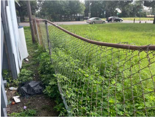
Chain Link Fence Damage Example
