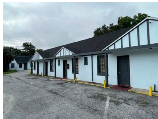
Faded Parking Stall Striping
