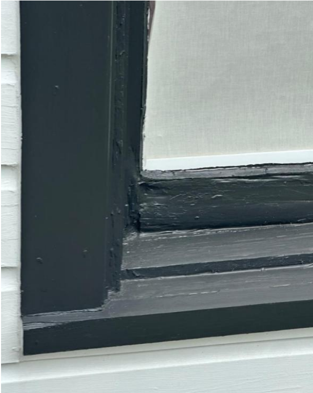
Deteriorated condition of the windows
