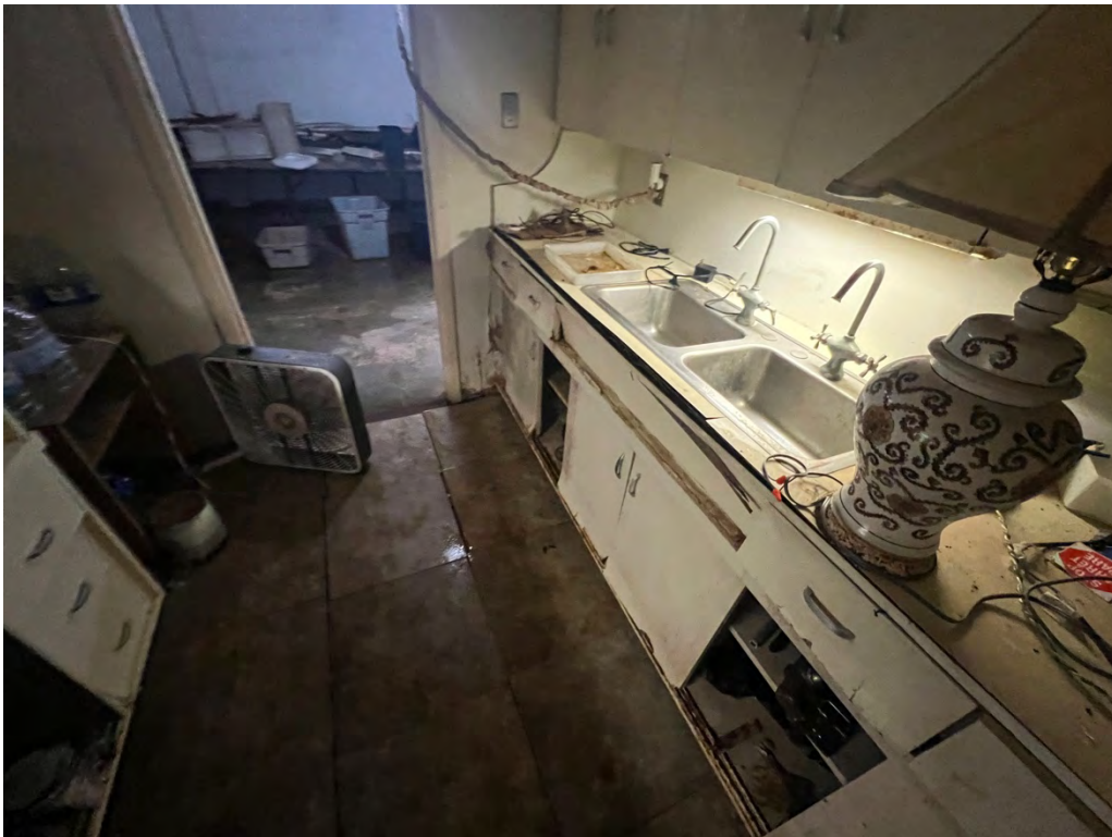
(13) Interior View – standing water, rot, moisture.
