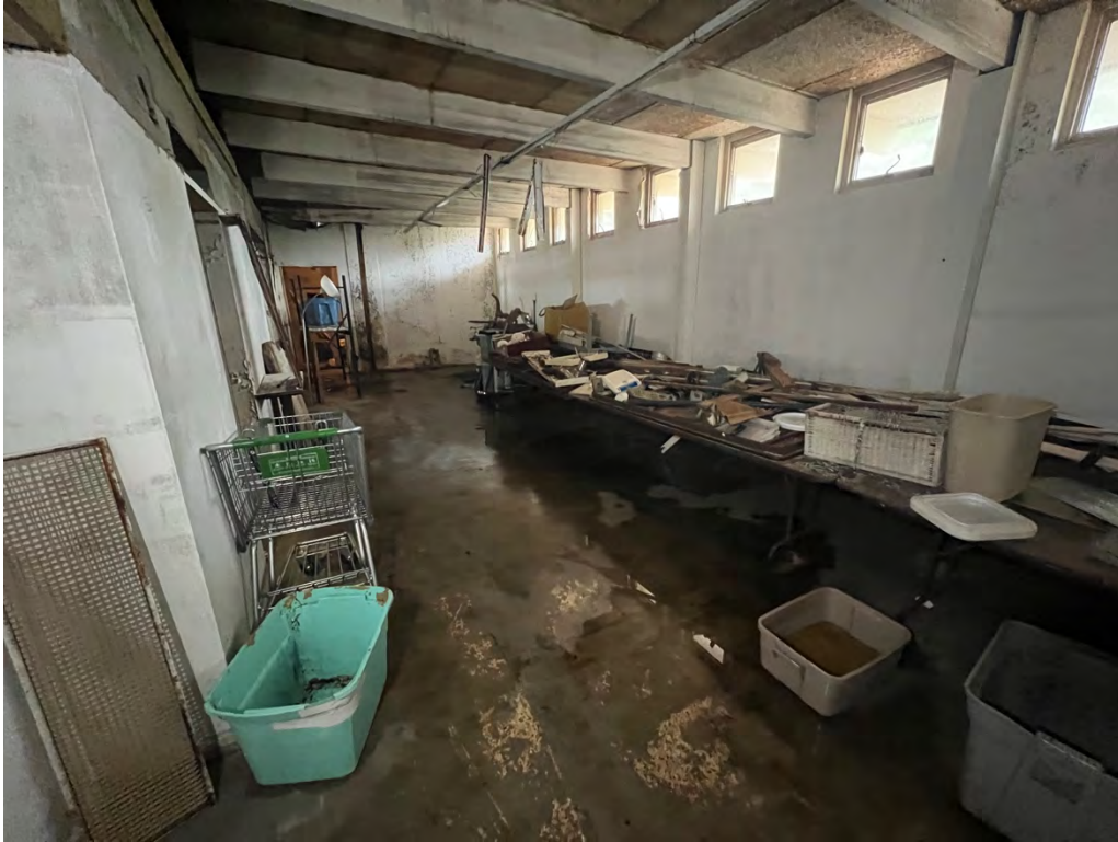
(14) Interior view – standing water, mold, leaking ceiling.
