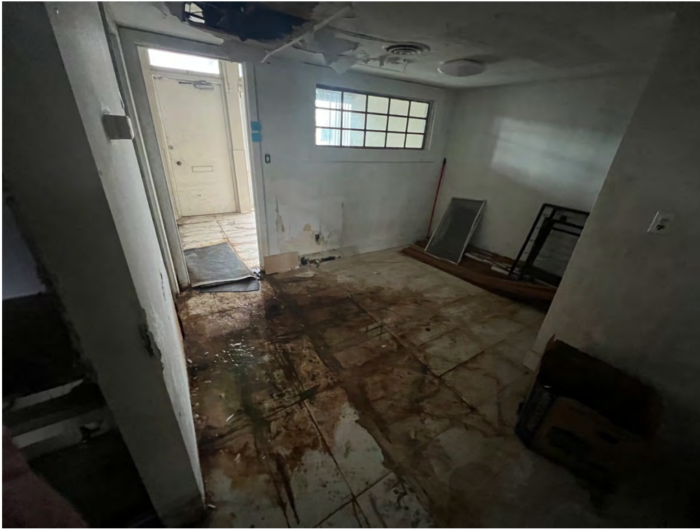
(7) Interior view – standing water, deteriorated ceiling.
