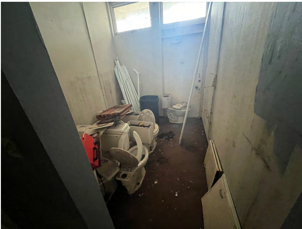
(15) Interior view – accumulated debris, infestation, mildew.
