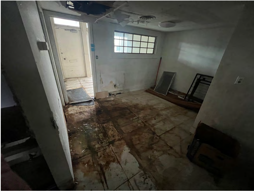
(7) Interior view – standing water, deteriorated ceiling.
