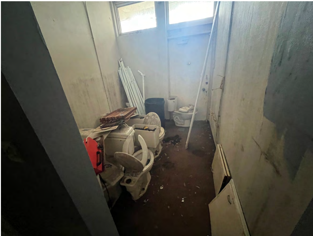
(15) Interior view – accumulated debris, infestation, mildew.
