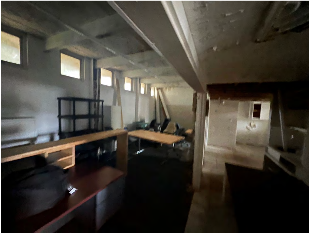
(12) Interior view – accumulated debris, deteriorated ceiling.
