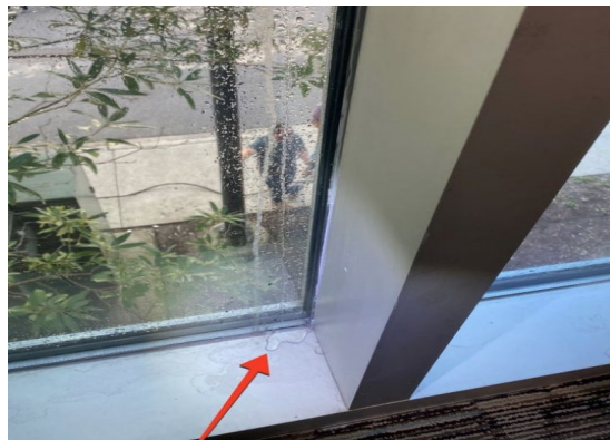
Confirmed water intrusion
