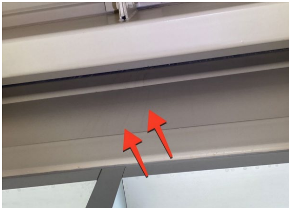
Confirmed water intrusion
