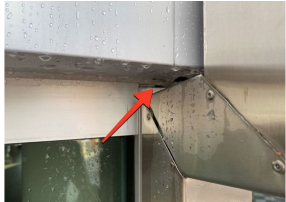
Confirmed water intrusion
